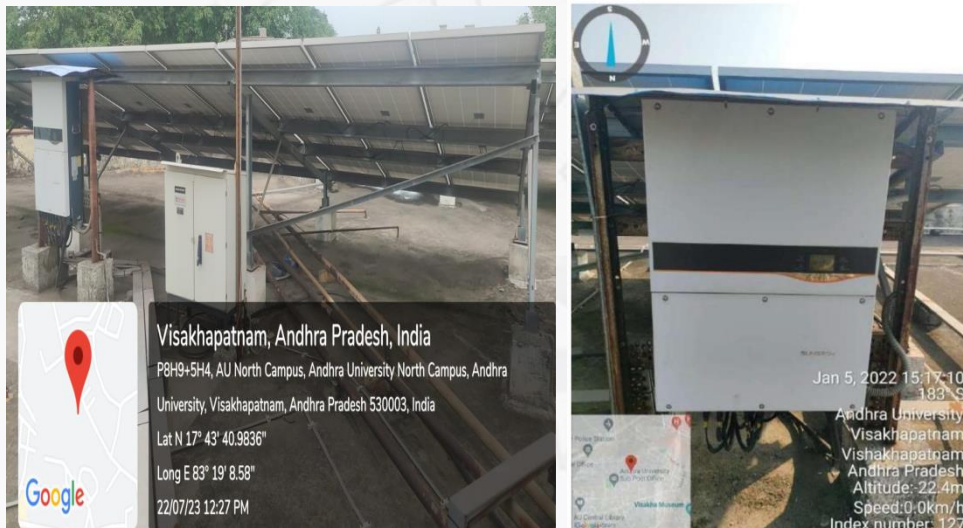
Solar Energy Panels
